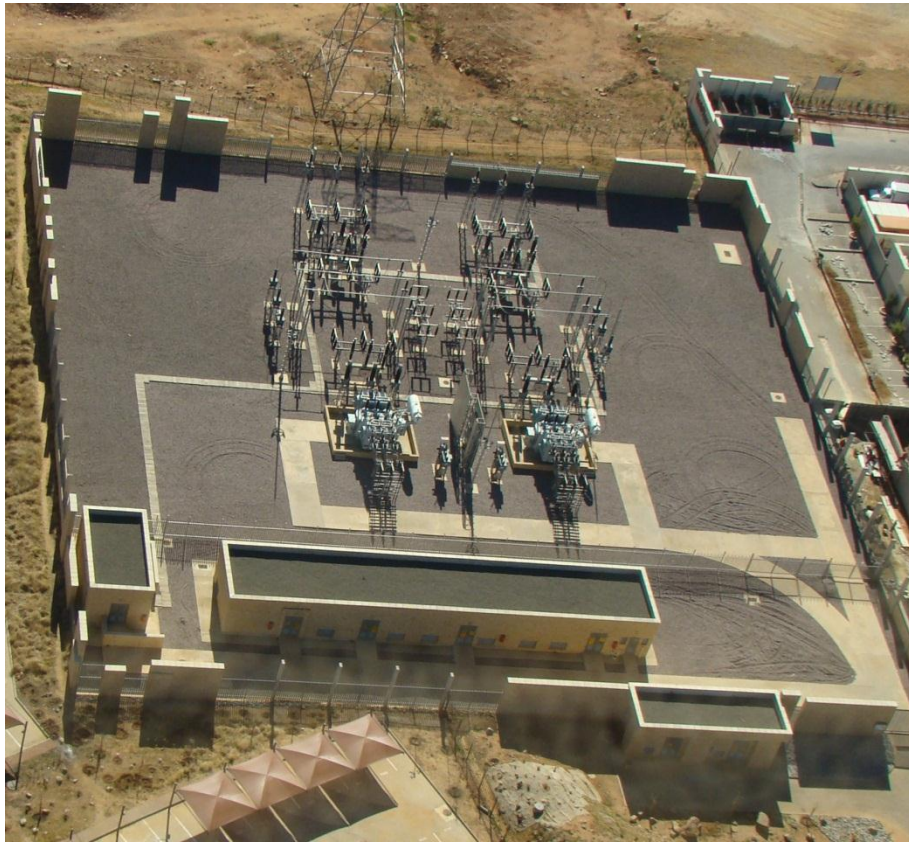
Figure 7 – Typical 132kV substation
