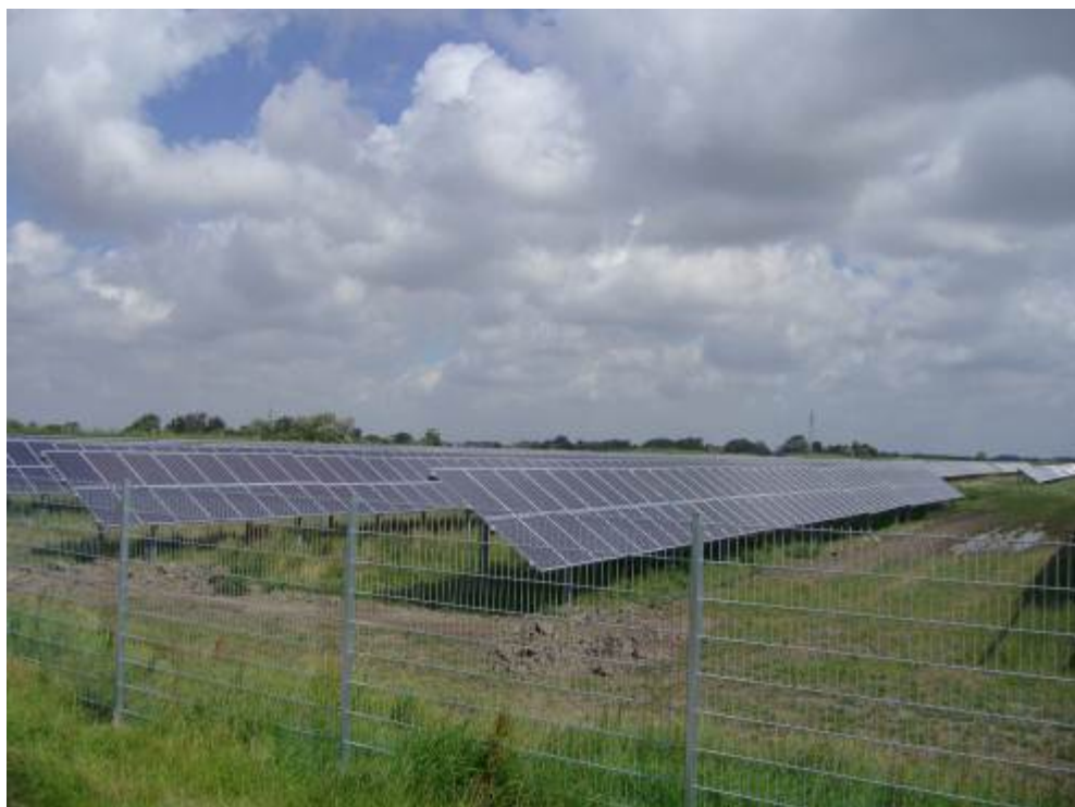
Figure 3: Photo showing an example of a PV facility and associated infrastructure.
