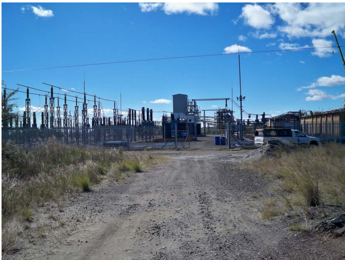
Figure 14: View Spruitfontein substation from the access road to the site
