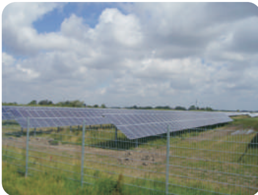
Figure 1: Photo showing view of photovoltaic panels from ground level
