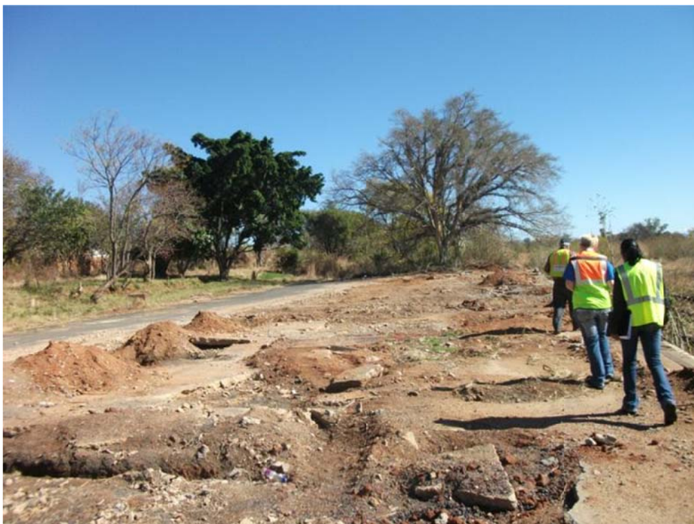
Figure 4: Photo of the area where the old Barberton railway station building occurred, which has been demolished
