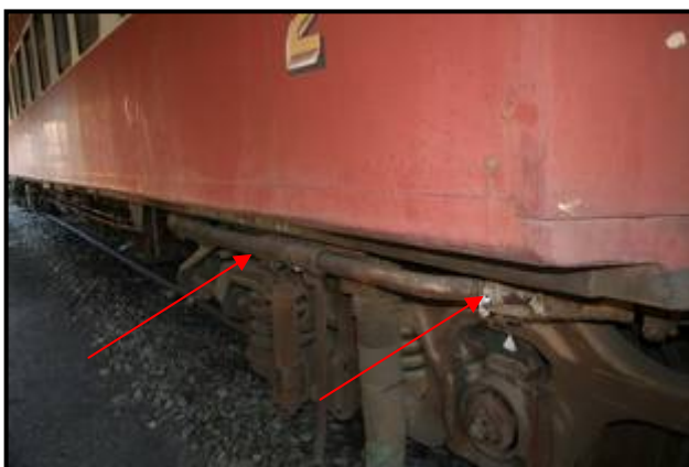
Figure 18: Ladanna – Asbestos Rope on Steam Pipes
