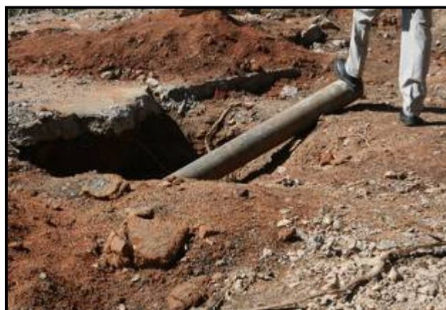
Figure 13: Barberton – Asbestos Cement Pipe from demolished building
