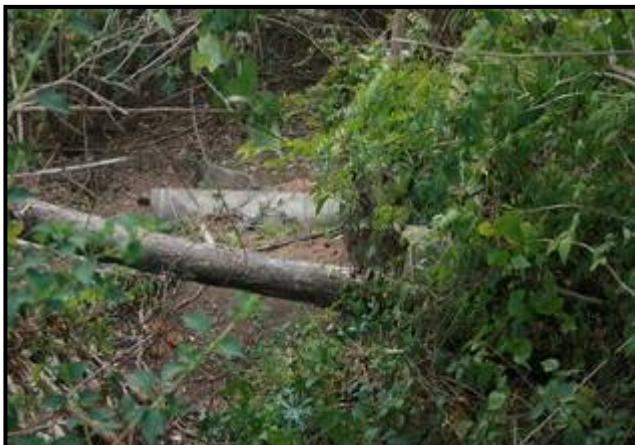
Figure 2: Nelspruit – Asbestos Cement Pipes
