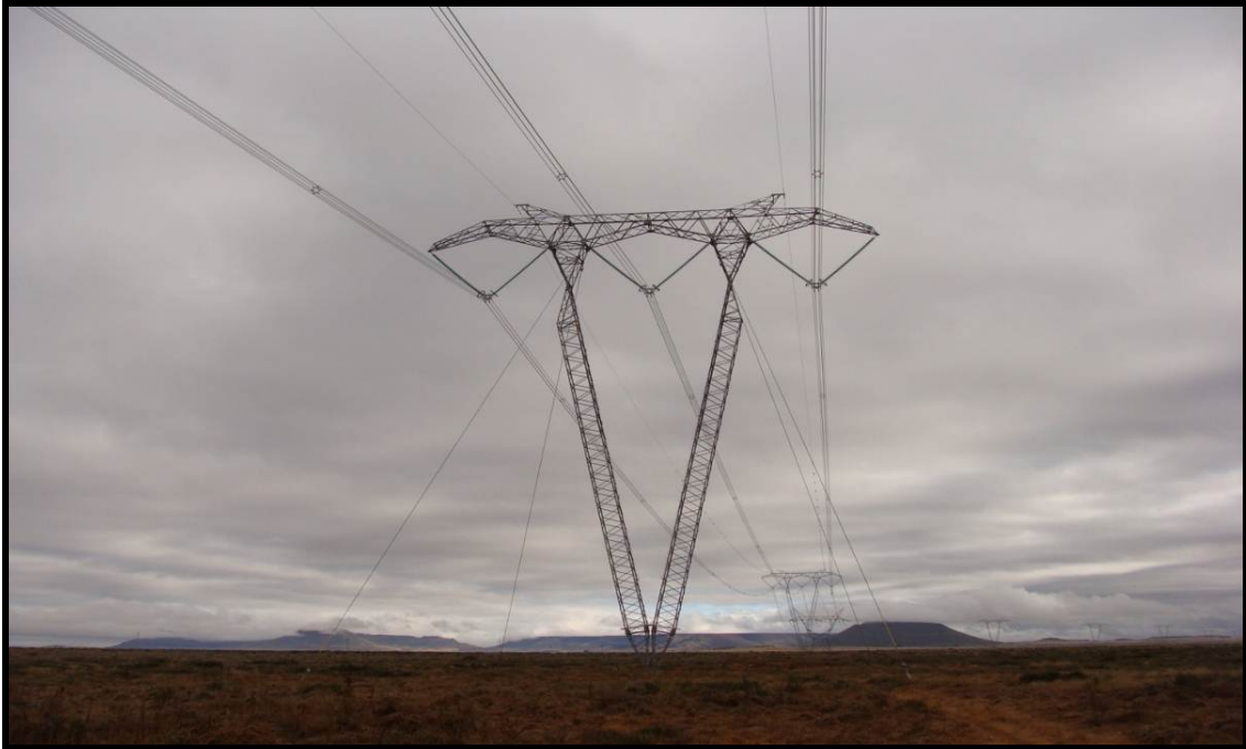
Photograph: 1.2: Existing Eskom Hydra MTS-Behrshoek 132 kV power line that traverses the site
