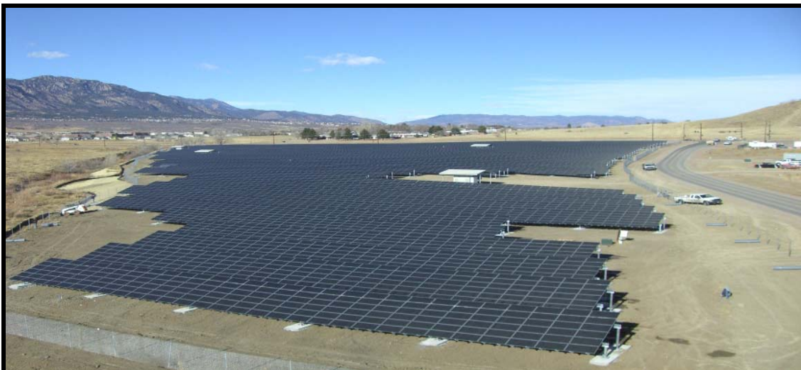
Photograph 1.1: Example of Photovoltaic array (Source: www.wapa.gov )
