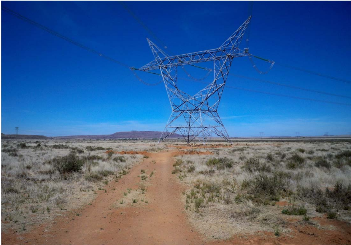
Figure 7: View of the Hydra-Perseus 765 kV power line that crosses the site.
