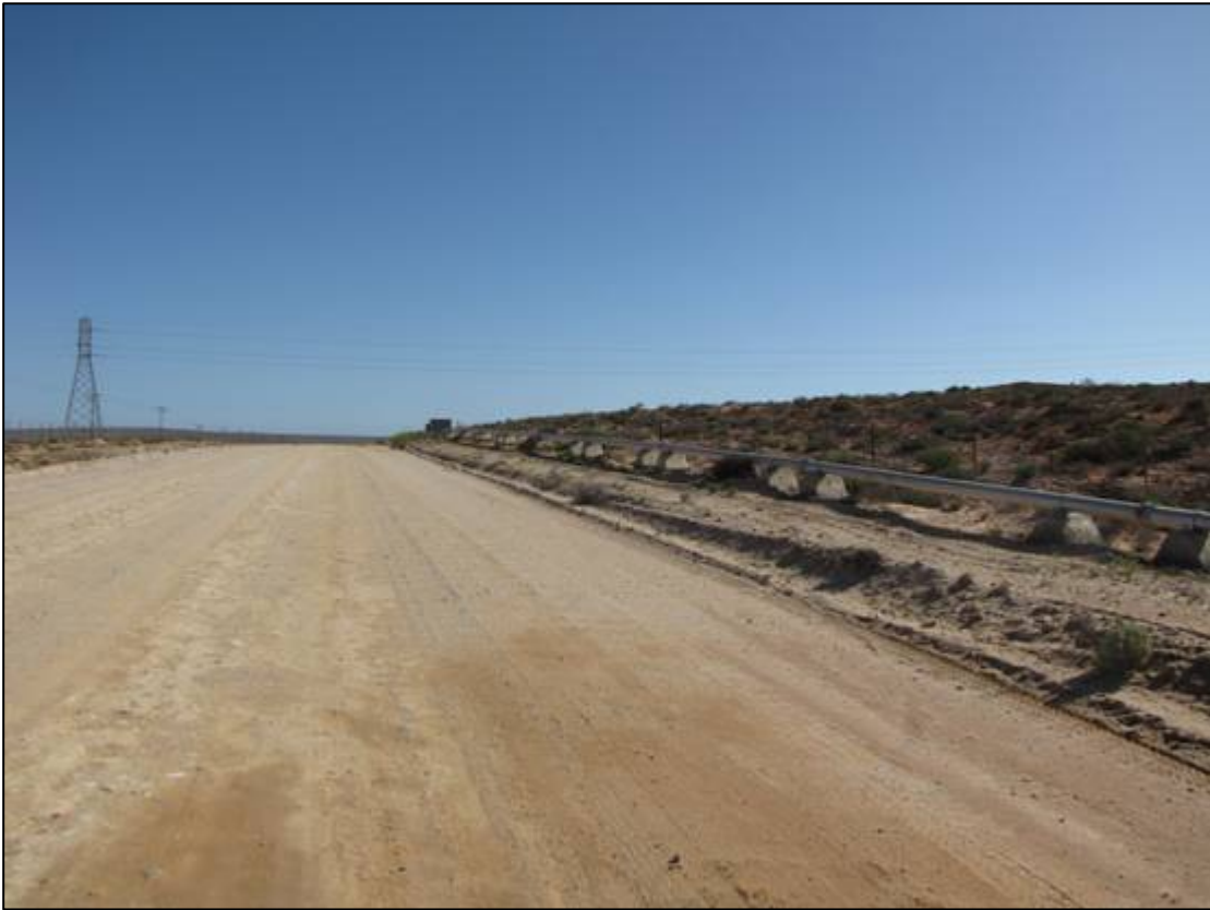
Figure 2: The R355 approaching Kleinsee with 220kV power lines crossing the road (in the vicinity of the Gromis Substation).
