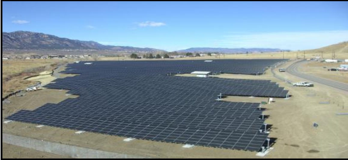
Photograph 1.1: Example of Photovoltaic array (Source: www.wapa.gov )
