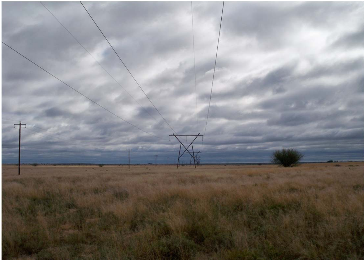
Figure 3: Electrical Infrastructure that crosses the site.
