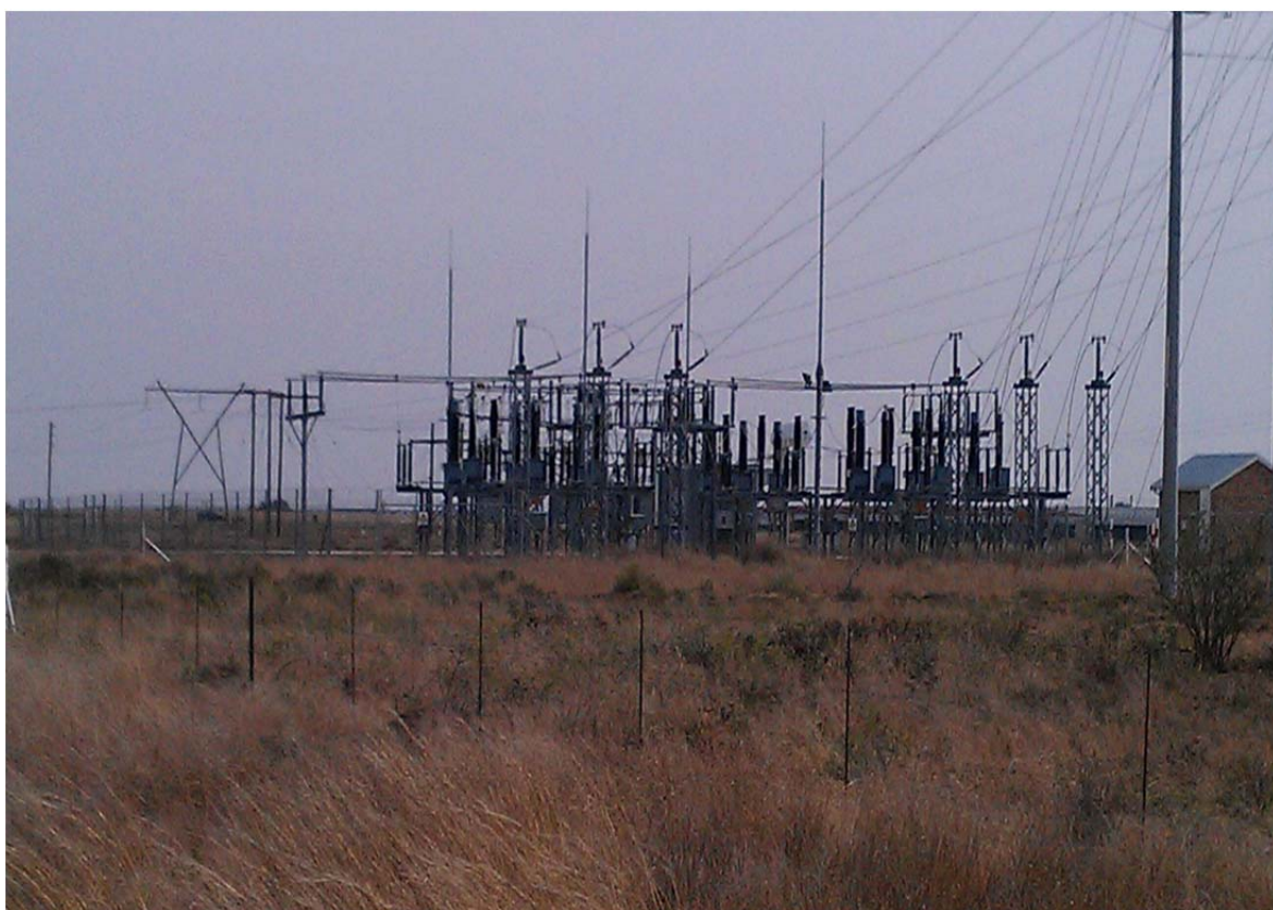
Figure 9: Closer view of Ritchie substation
