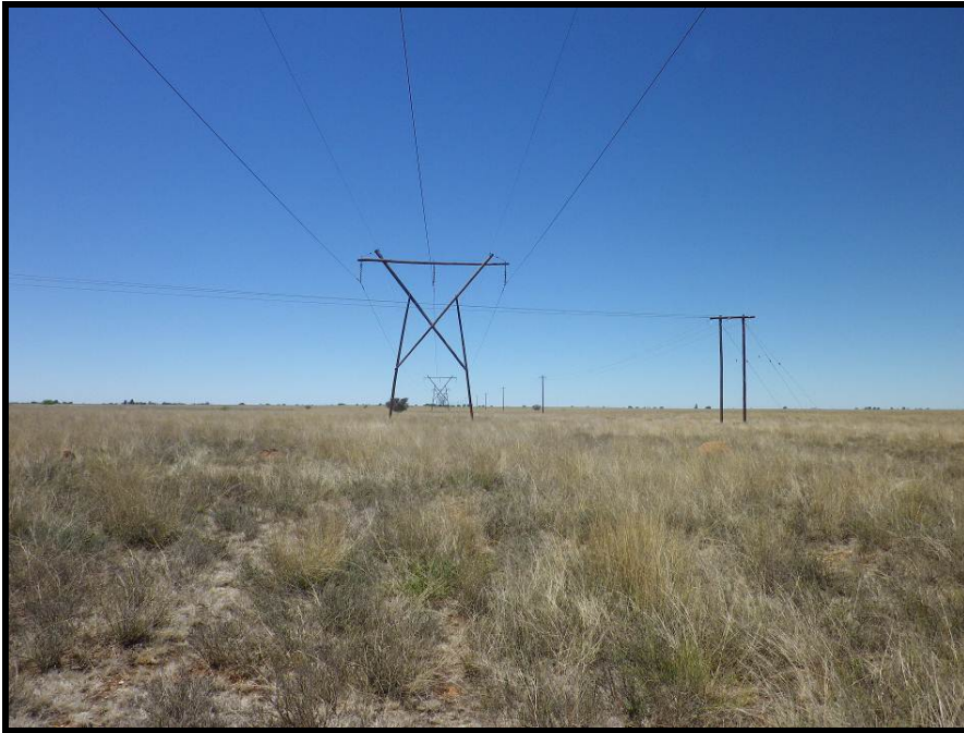
Photograph 2.4: View of power lines running across the northern section of the site
