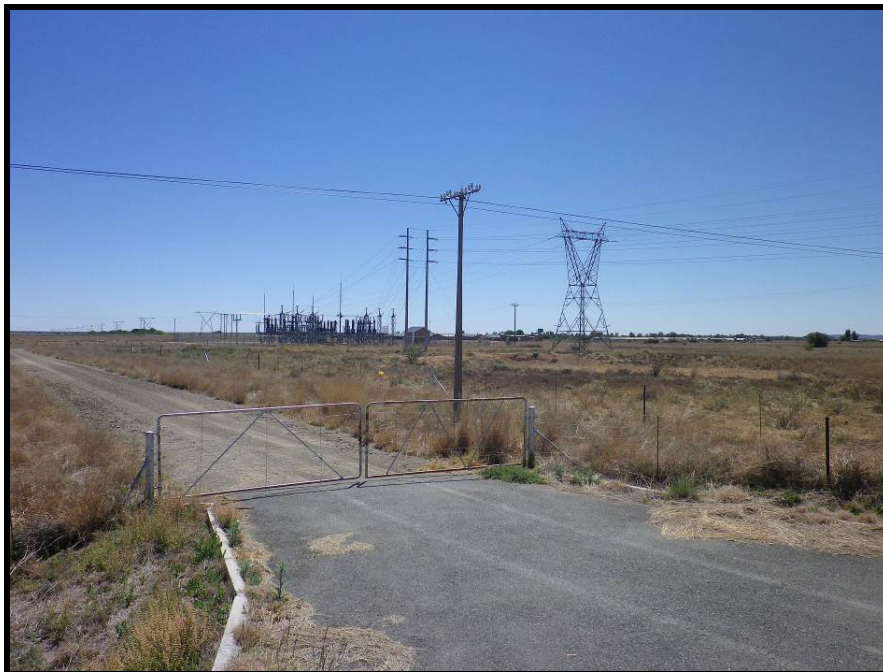
Photograph 2.3: Ritchie substation with chicken broilers in the background
